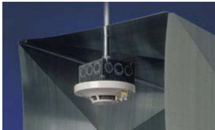
Top Mount in Ventilation Shaft
